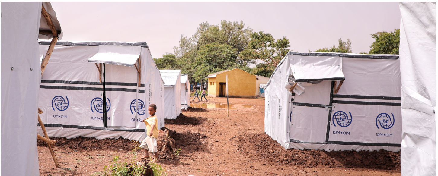
IOM and partners are building shelters in an IDP site in Shire, Tigray Region. Photo: IOM/Kaye Viray
