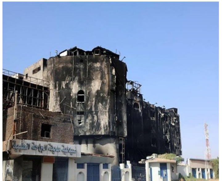
DESTROYED HOSPITAL IN BAHRI, KHARTOUM - APRIL 2025 IOM
