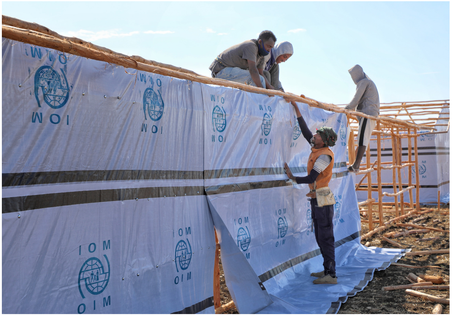
IOM and partners are building shelters in Sabacare 4 IDP site in Mekelle, Tigray Region. Photo: IOM/Kaye Viray
