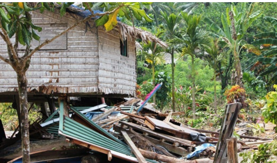
Damage at Nela Village, Temotu Province, Solomon Islands. A magnitude 7 aftershock occurred off the Santa Cruz Islands in early February 2013– less than three days after the initial magnitude 8 quake and tsunami impacted on 25 communities. © Matt Anderson/DFAT, 2013
