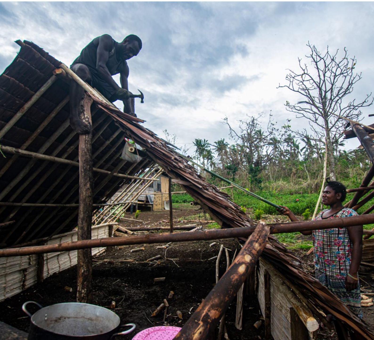
Families building a new kitchen beside the damaged house. Vunavose, South Santo, Vanuatu, April 2020, © UNICEF/UNI324720/Shing
