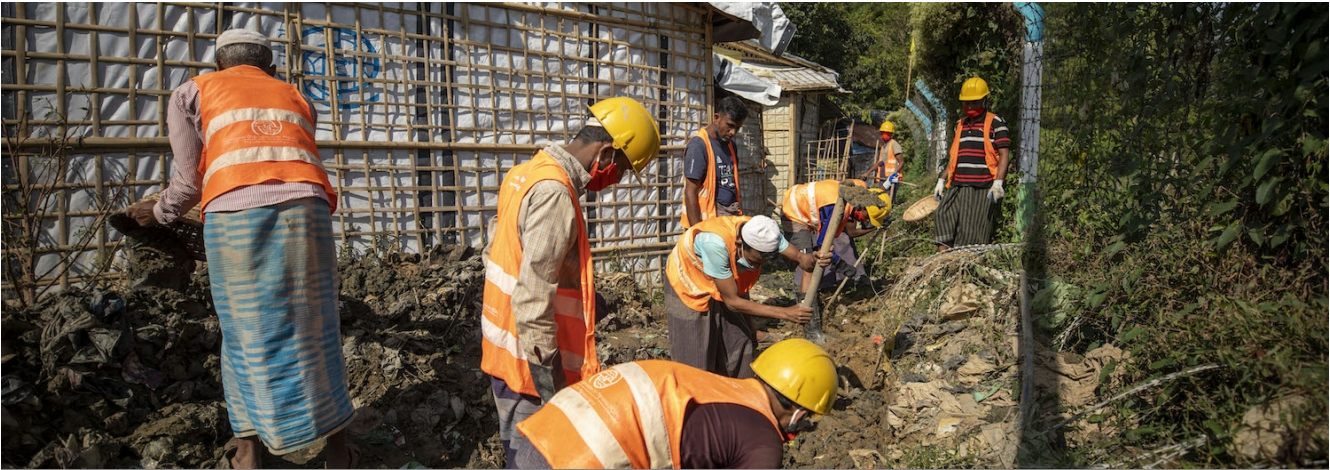
Refugees working on a drainage to ensure the flow of storm water. © IOM Bangladesh 2022 / Abdullah Al Mashrif
