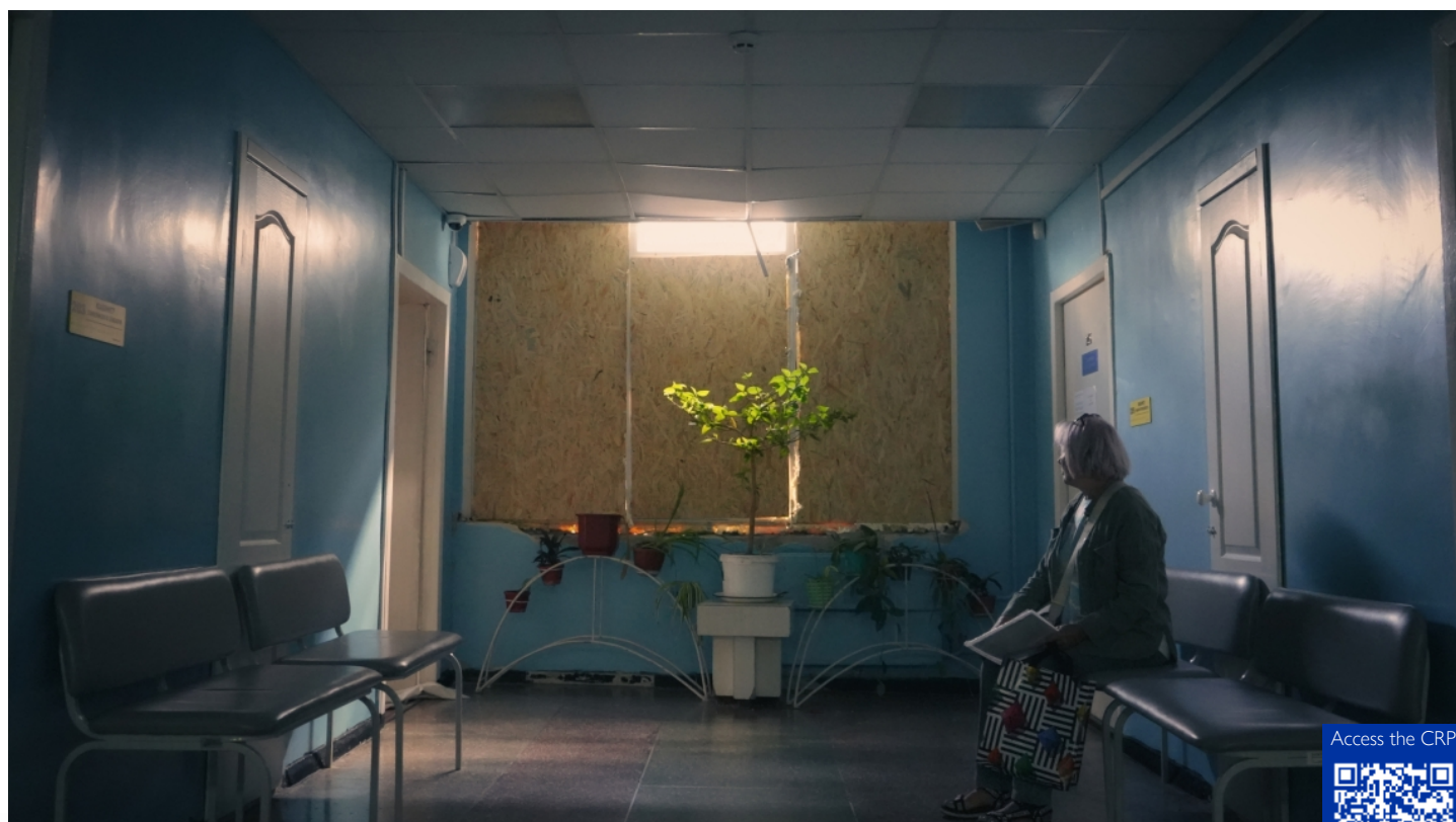
A patient at a hospital in Kharkiv waits outside the doctor's office, glancing at the window damaged from a blast wave during an attack in June 2024. © IOM Ukraine/Anna Tsybko
