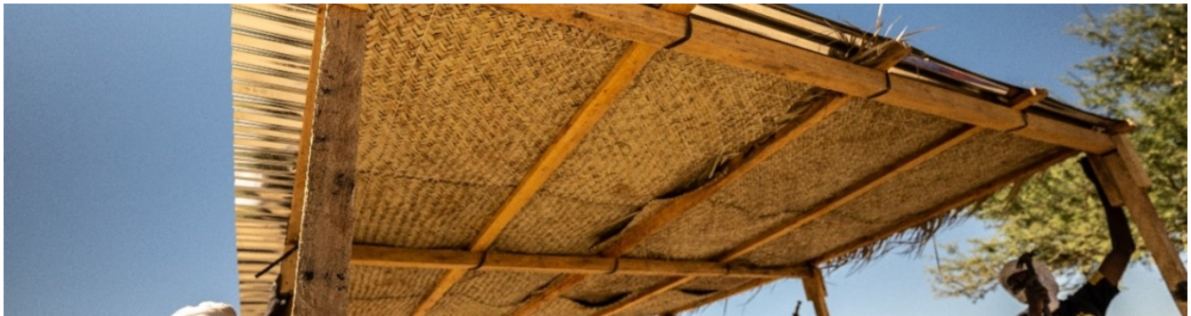
Lake Chad Province, men working on shelter construction. © IOM Chad / Andrea Ruffini, 2020
