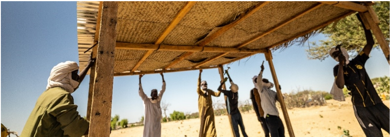
Lake Chad Province, men working on shelter construction. © IOM Chad / Andrea Ruffini, 2020
