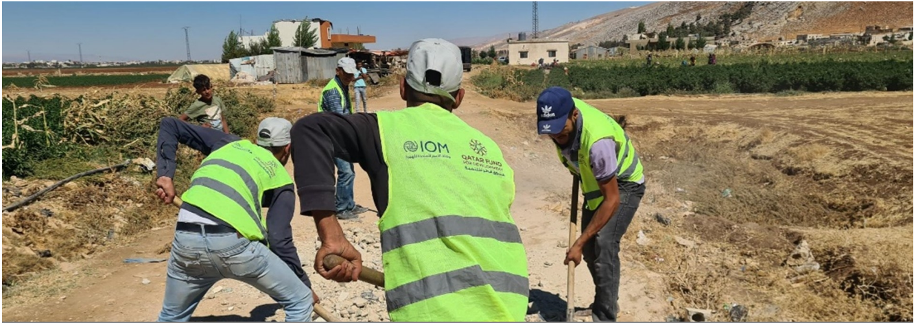
Cash for Work beneficiaries rehabilitating a road in Faour, Bekaa. @ IOM Lebanon 2022.
