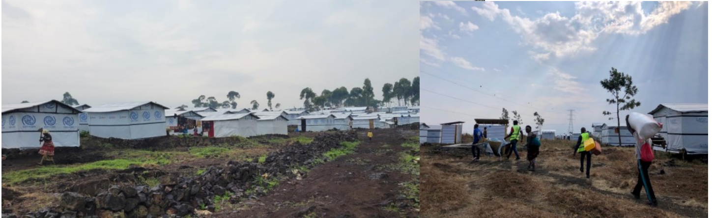
Shelters constructed by IOM and support to transfer operations organized by CCCM teams, Rusayo 2 and Bushagara sites, North Kivu © IOM 2023
